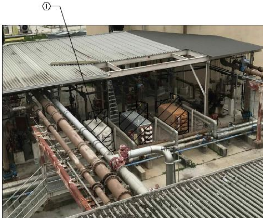
DESCRIPTION: AERIAL VIEW OF PUMP STATION NO. 3 HIGHLIGHTING ALL THREE HEAT EXCHANGERS. PUMP STATION NO. 4 IS TYPICAL OF PUMP STATION NO. 3 HOWEVER THE LAYOUT IS MIRRORED.
