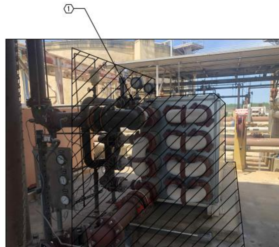
DESCRIPTION: TYPICAL FRONT VIEW OF HEAT EXCHANGER HIGHLIGHTING THE SLUDGE AND HOT WATER INLET AND OUTLET CONNECTIONS.
