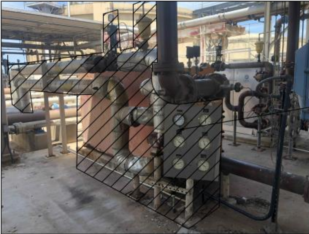
DESCRIPTION: TYPICAL SIDE VIEW OF HEAT EXCHANGER HIGHLIGHTING HOT WATER PIPING AND EQUIPMENT AS WELL AS GENERAL INSTRUMENTS.
