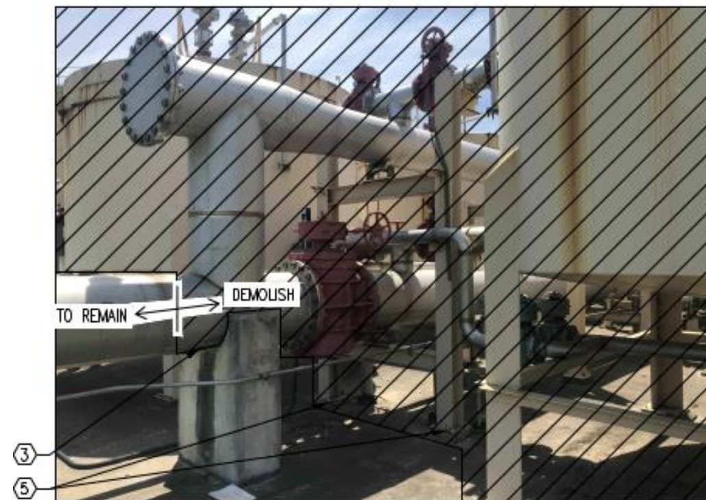
DESCRIPTION: VIEW OF IRON SPONGE PIPING FACE WEST. THE HEADER SHOWN RUNS WEST TO THE GAS FLARE STATION.
