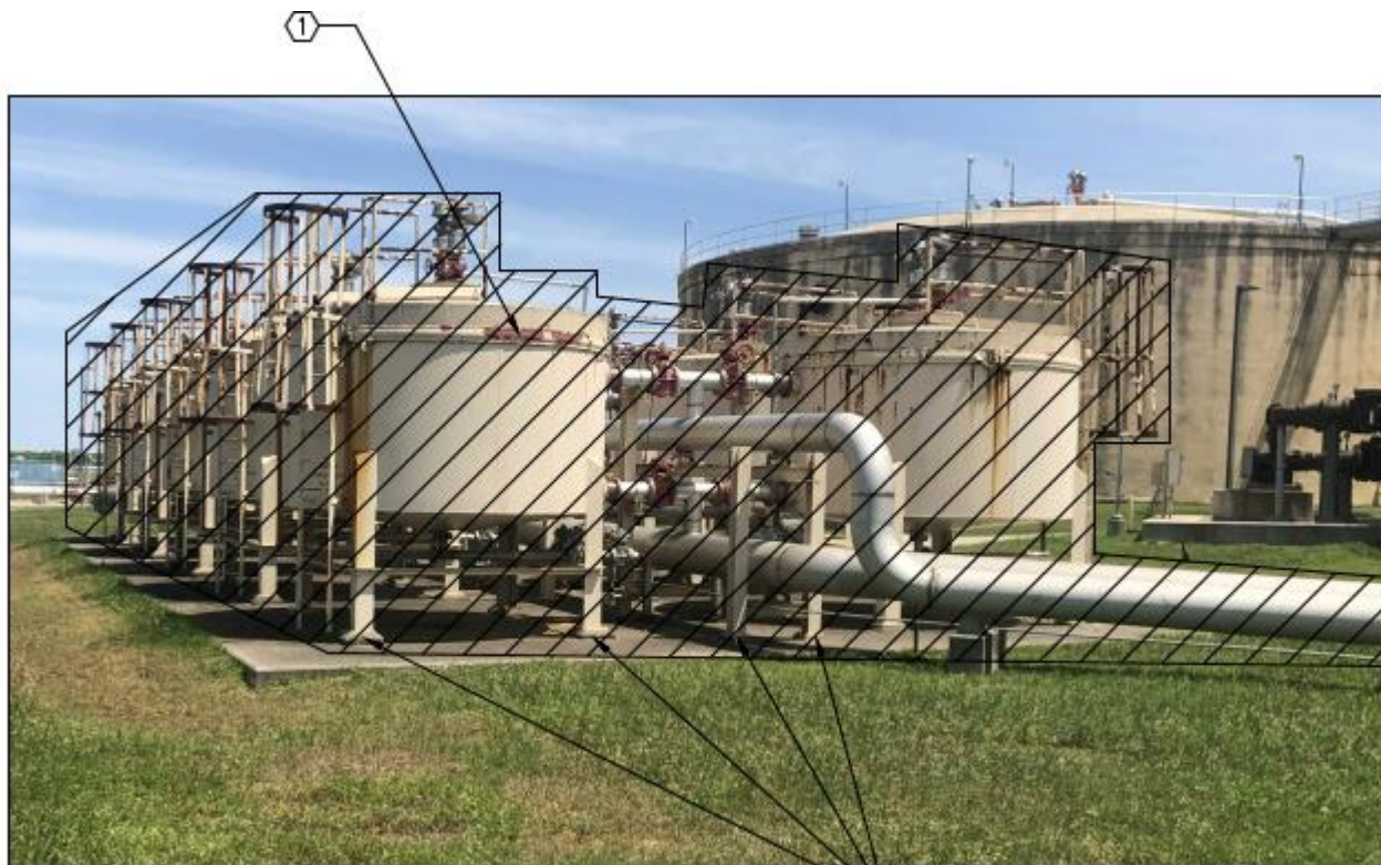
DESCRIPTION: VIEW OF IRON SPONGES FACING EAST.
